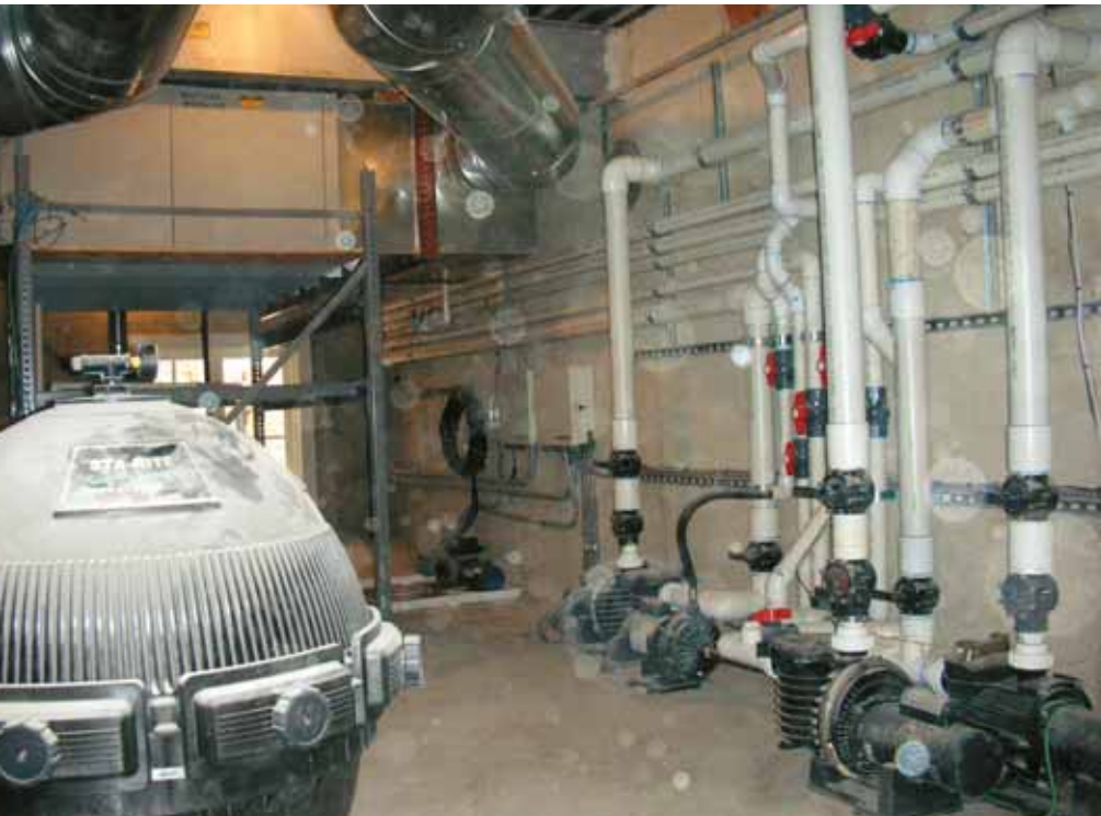
ABOVE: Below the pool patio level, HVAC and dehumidification systems had to share space with the pool mechanical systems. The pool piping and HVAC venting had to be installed in coordinated phases for each to be optimized and operate efficiently.
